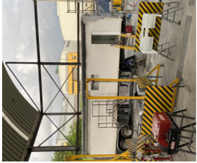
NINOX production floor with the semitrailer under equipment installation. In the foreground, the electrical generation system and NINOX precision welding equipment.
